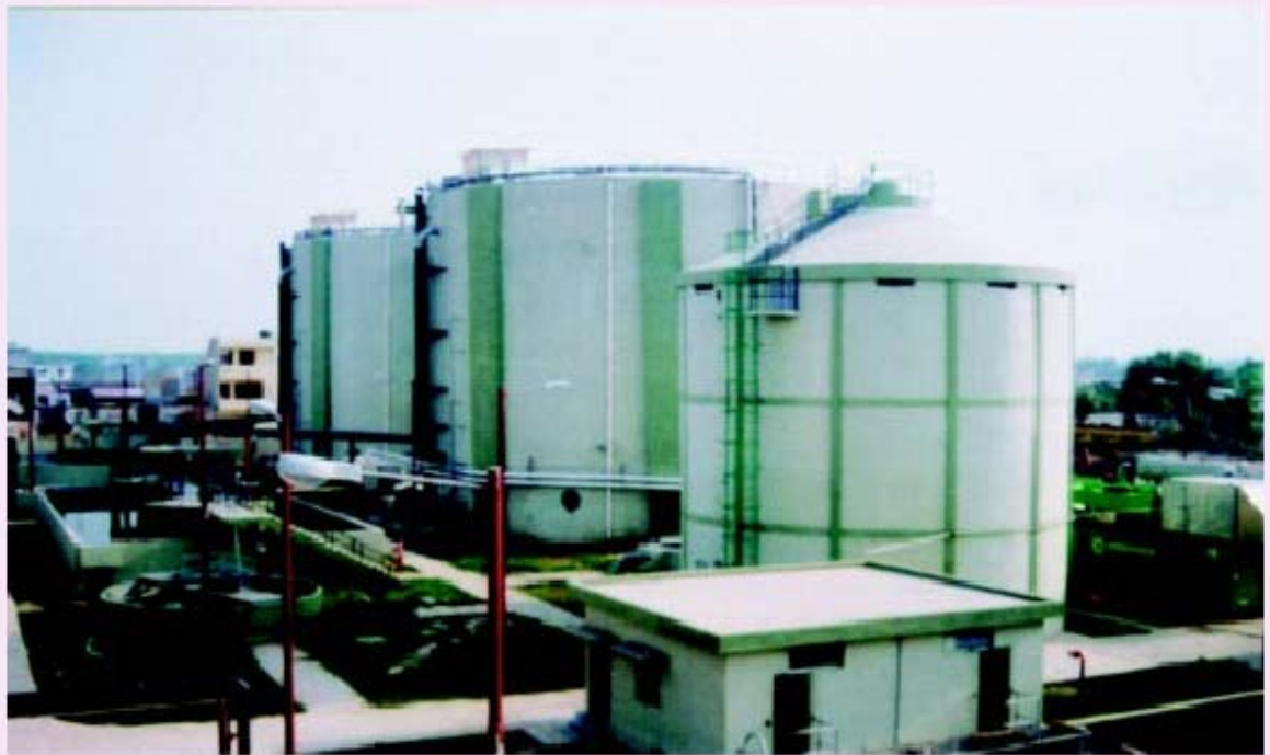
1-MW power project based on cattle dung at Haebowal Dairy Complex, Ludhiana, Punjab
