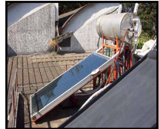
Test Facility for thermosyphon systems
