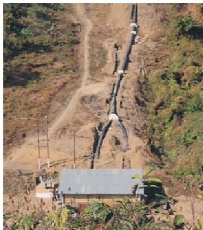
200 kW Chizami village, Nagaland
