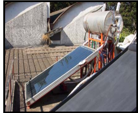
Test Facility for thermosyphon systems
