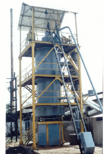
Updraft Gasifier Steel re-rolling Raipur
