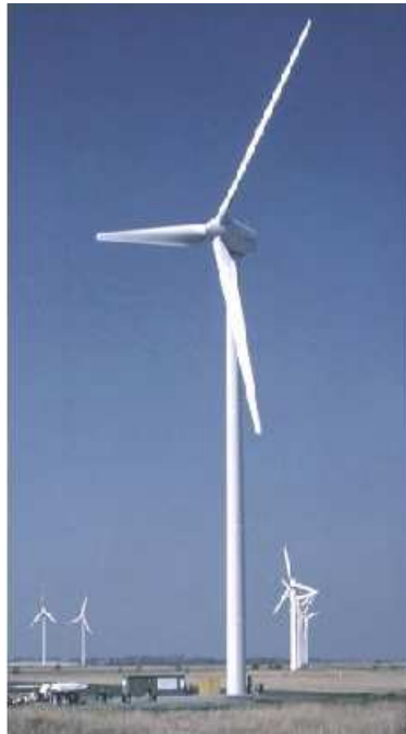
Fig. 1. Horizontal-Axis Large Wind Turbine (Courtesy: GE Energy)
